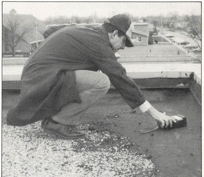
The smaller, hand-held model registers moisture infiltration by indicating variances on a meter.
