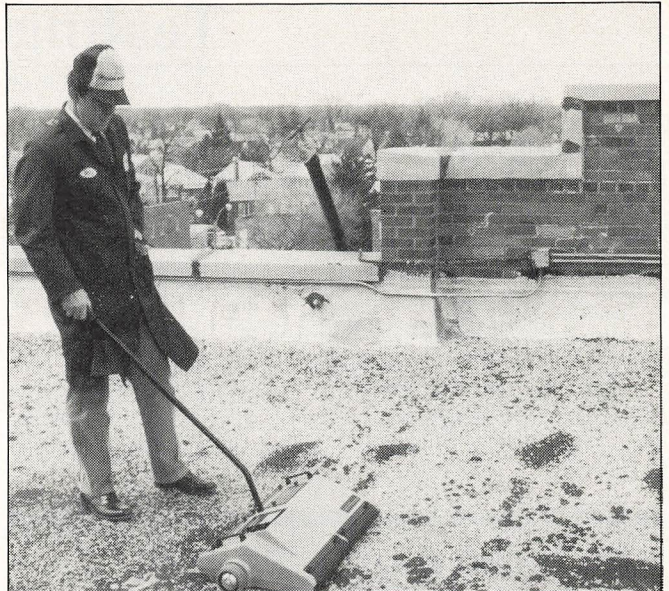
The larger electric capacitance moisture detector rolls over a roof area emitting tones when passing over a saturated area.
