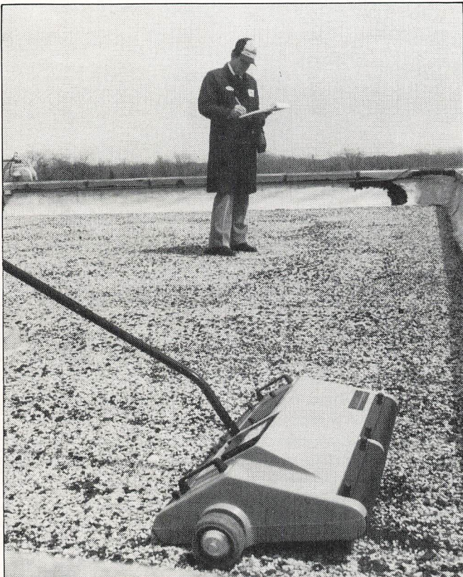
Promen plots out a roof, indicating those areas where moisture may have infiltrated.
