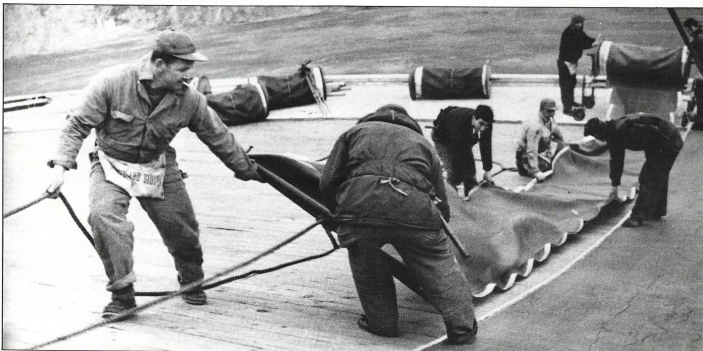
Workmen hold on to ropes to keep from falling off the ice arena's roof as they pull neoprene membrane into place.
