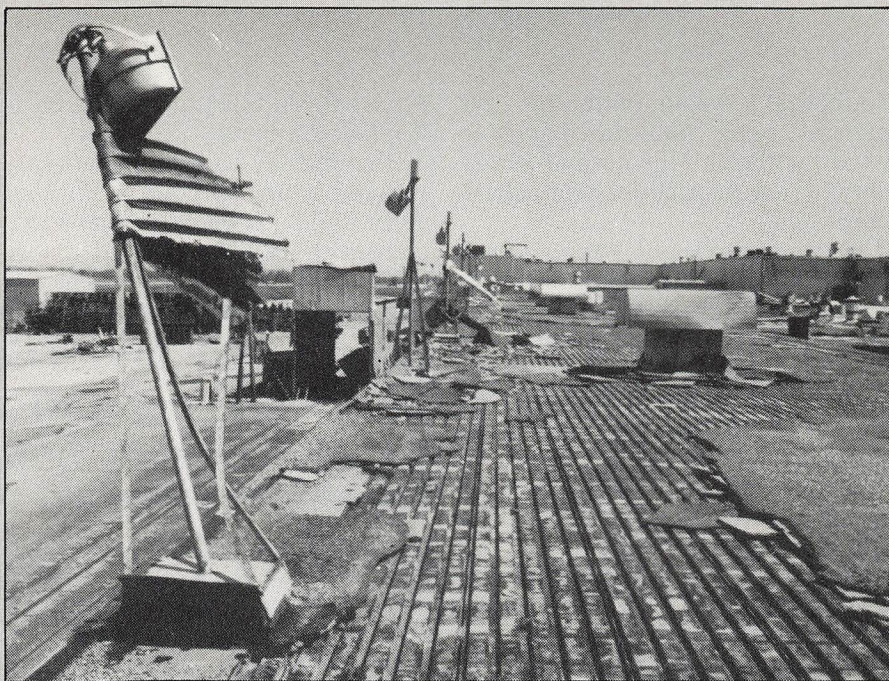
A Granite City, Ill. tornado rips apart the Smith Corp.'s roof.
