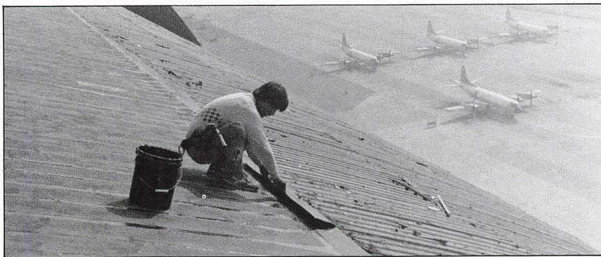
A workman applies tapered edge strips to the edge of Hangar One's roof.
