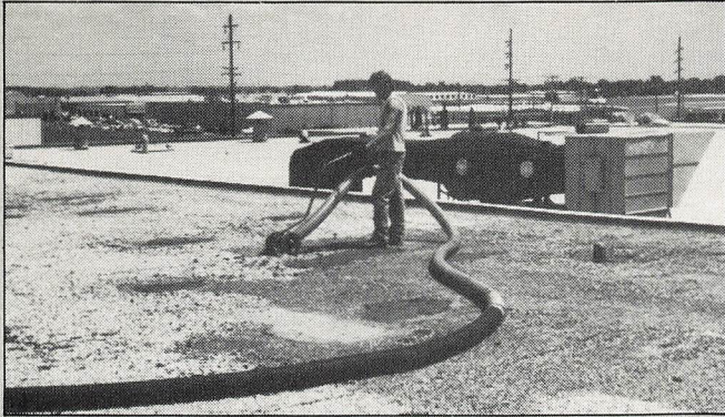
The old roof is prepared for an overlayment of single ply by vacuuming off the old roof aggregate.
