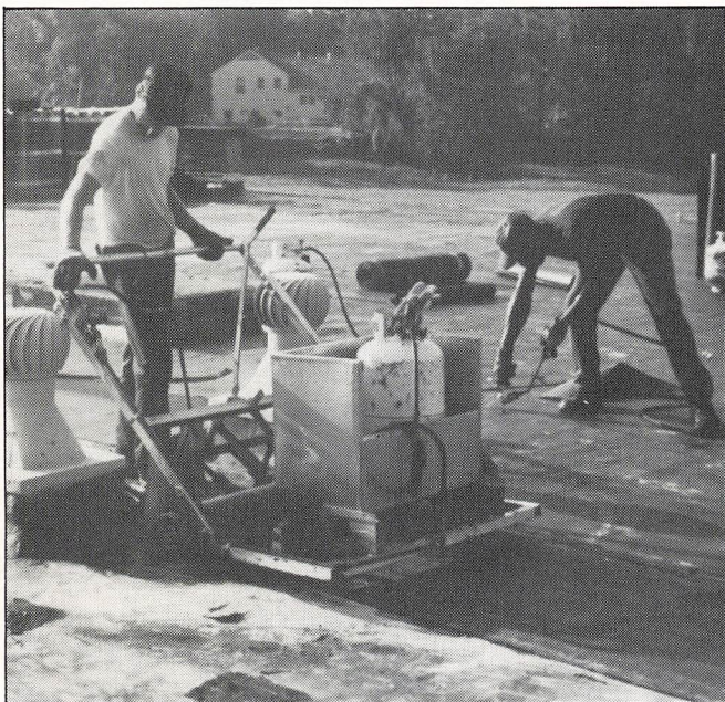
Derbigum, a modified bitumen system from Owens-Corning Fiberglas, is torched on to one of eight schools in the Shawnee Mission, Kansas School District.
