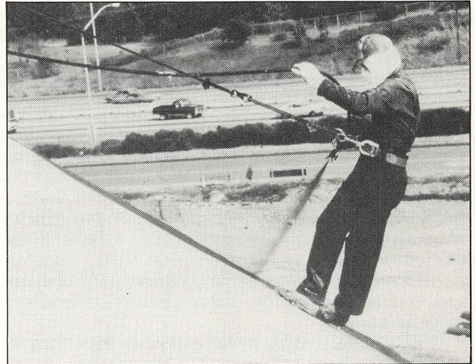
Application of sprayed-in-place polyurethane foam on the Tacoma Dome, Tacoma, Wash. (Photo courtesy of United Foam Contractors Association)
