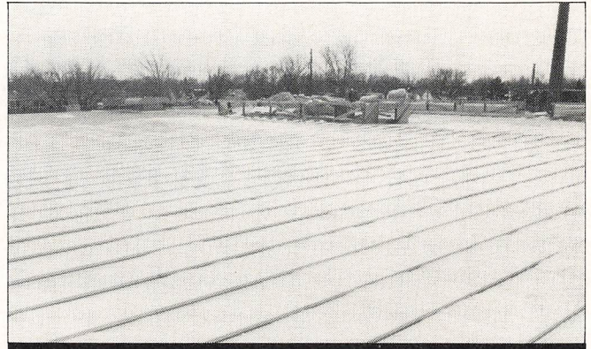
Step Seven — The school can expect years of maintenance-free performance from the standing seam metal roof. The re-roofed area totaled some 25,000 sq. ft.
