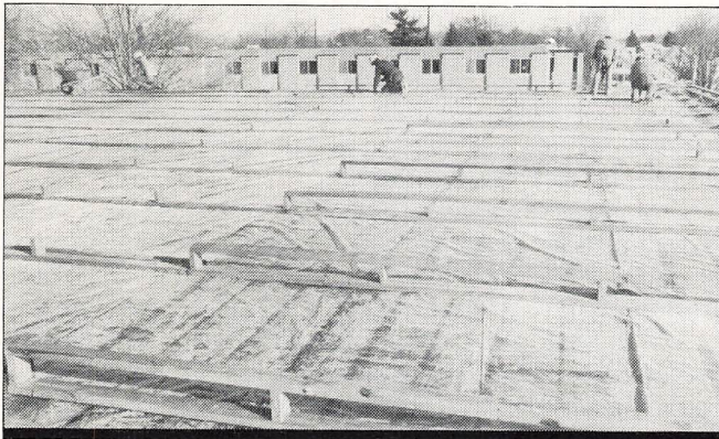
Step One — The original built-up roof on the field house was removed down to the decking. Contractors installed a 6 mil polyethylene vapor barrier and a lumber substructure to give the new roof a slight pitch for better drainage.
