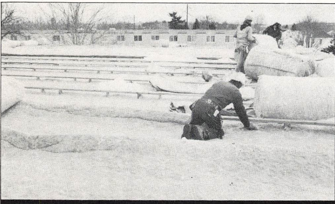
Step Two — Installers placed two layers of 3/4" fiber glass bat insulation between substructure members.
