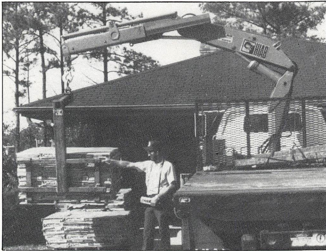
HIAB 650 hydraulic crane with proportional remote control system has helped John McDaniel Wholesale Supplies, Inc., of Atlanta, Ga., double on-site deliveries of roofing materials.
