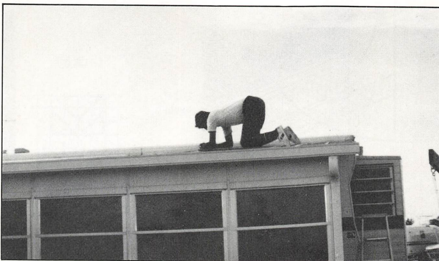
NRCA Officers at Work Dep't: That's NRCA VP Bob Bubenzer checking for a leak in the metal roof covering his Florida home. And we wondered where all that know-how came from.
