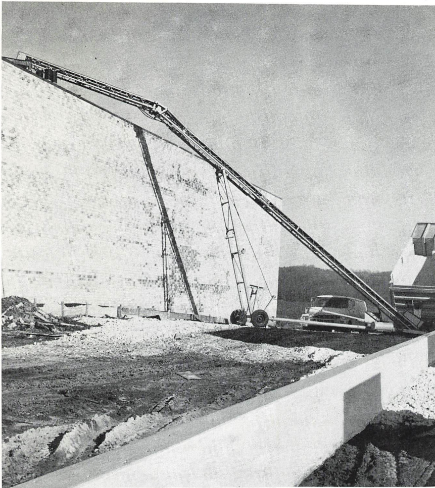
Articulating boom lets Morgen Roofers Conveyor work at an angle within limited access on F. A. Taylor job in Maryland.
